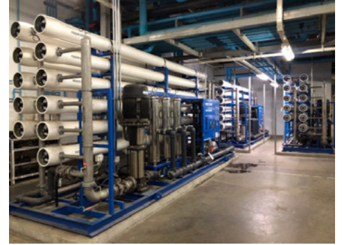
RO membrane facility
